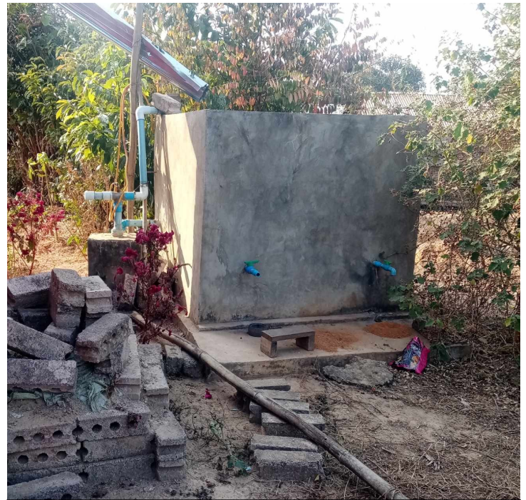
A generator is needed to run the pump to supply water to the village. The government has shut off electricity.
