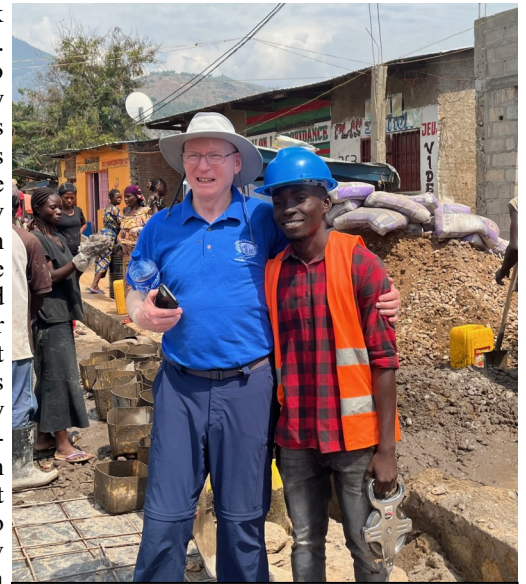
Bill and Washikala, one of the CCC orphans who went to university on a Global Outreach scholarship and became a civil engineer. He is working hard on the road project.
